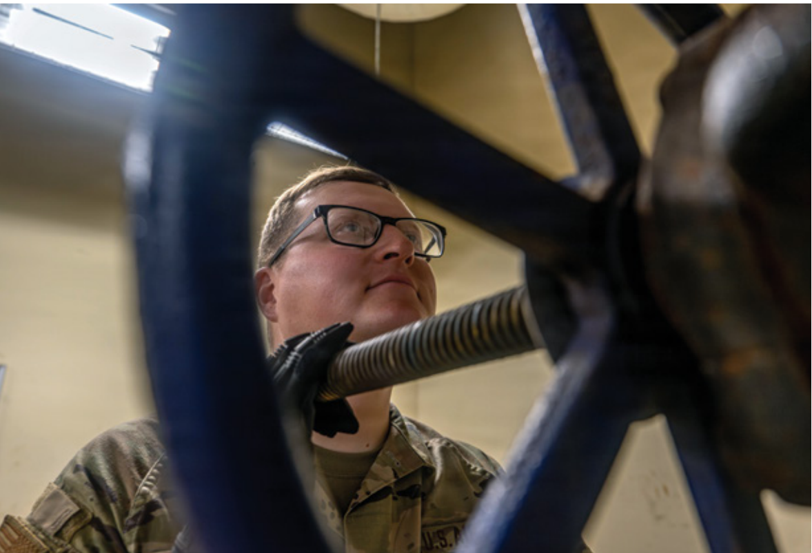
U.S. Air Force Tech. Sgt. Matthew Kramer, 8th Civil Engineer Squadron heating, ventilation, air conditioning, and refrigeration non-commissioned officer in charge, monitors water temperature gauges in HVAC infrastructure supporting base dormitories at Kunsan Air Base, Republic of Korea, July 16, 2026. (U.S. Air Force photo by Senior Airman Dylan Maher) ▲
