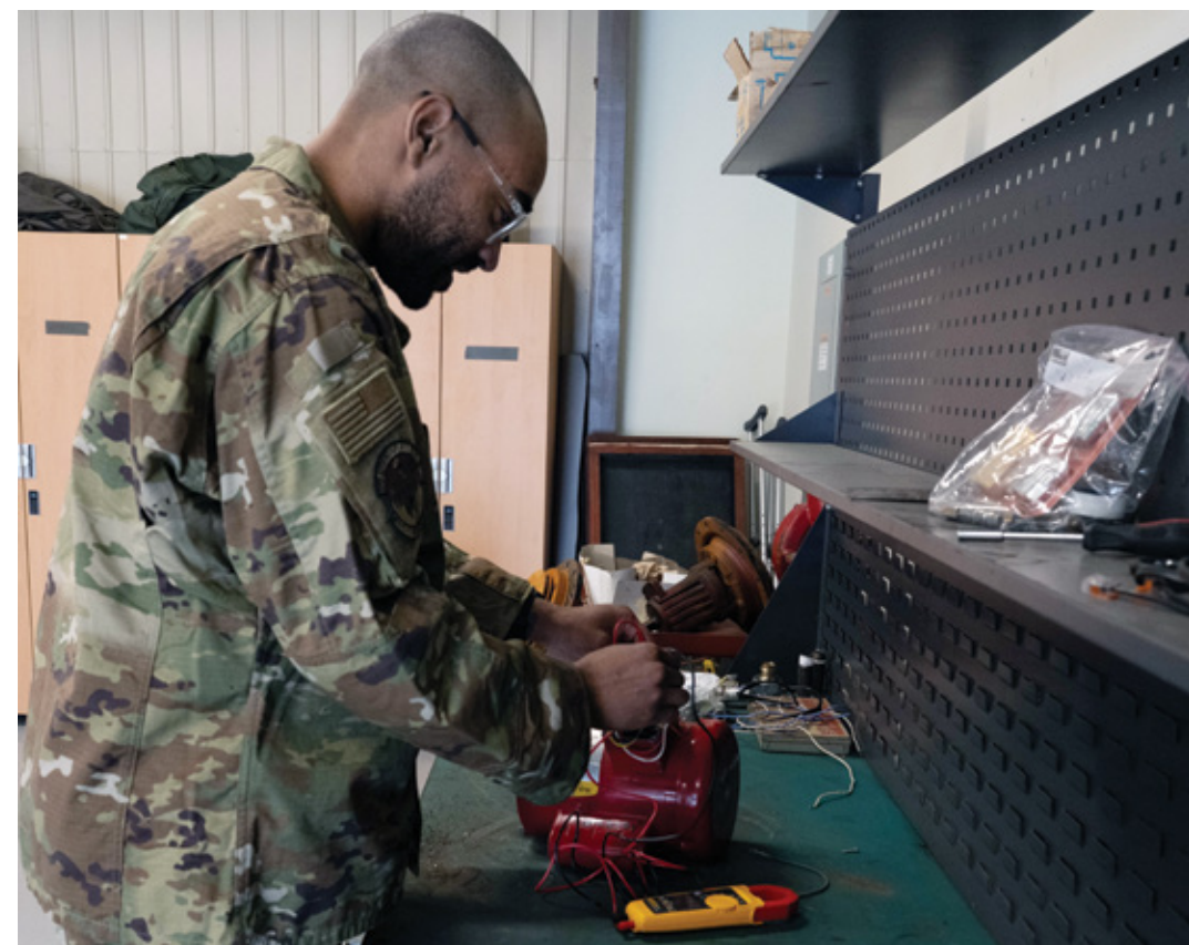
U.S. Air Force Staff Sgt. Tyrone Wilson, 8th Civil Engineer Squadron heating, ventilation, air conditioning, and refrigeration journeyman, checks wire continuity on a pump motor at Kunsan Air Base, Republic of Korea, April 30, 2026. Wilson was selected as the Wolf Pack's Pride of the Pack for the week of April 27 - May 1 due to his achievements within his career field and his impact on the readiness and well-being of the Wolf Pack. ▲
