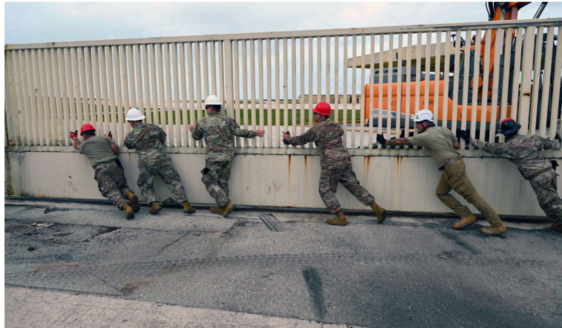
U.S. service members assigned to the 8th Civil Engineer Squadron, Marine Wing Support Squadron 174, Marine Corps Base, Hawaii and the Naval Mobile Construction Battalion, Chinhae, Naval Base, Korea, clear a crater as part of a joint-service Rapid Damage Repair training at Kunsan Air Base, Republic of Korea, March 23, 2026. ▲
