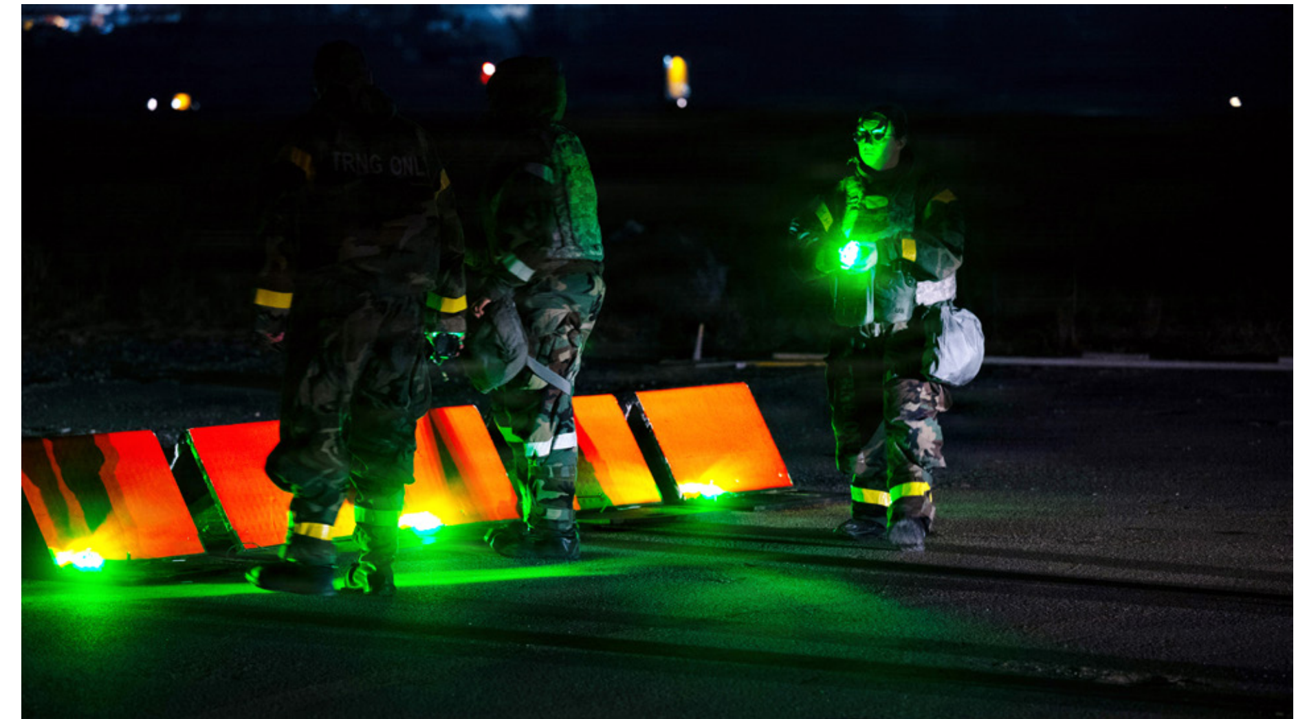
U.S. Air Force Airmen assigned to the 51st Operations Support Squadron and the 51st Civil Engineer Squadron place a lighting system on a minimum operating strip during exercise Freedom Shield 26 at Osan Air Base, Republic of Korea, March 11, 2026. The exercise demonstrated interoperability between two units to rapidly establish and operate a makeshift runway if the primary airfield is degraded or unusable. FS26 provides a demanding training environment designed to enhance combat readiness and response capabilities. (U.S. Air Force photo by Tech. Sgt. Desiree Ware) ▲
