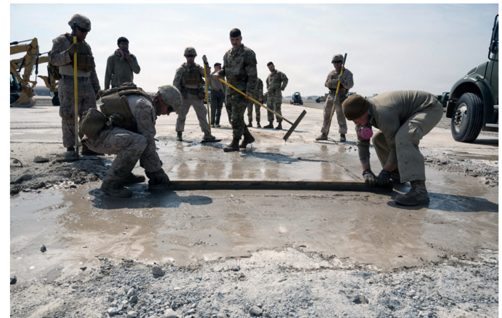
U.S. Marine Corps Lance Cpl. William Hayes, left, Marine Wing Support Squadron 174 combat engineer and Senior Airman William Johns, 8th Civil Engineer Squadron pavement and equipment operator, level out rapid set concrete during a joint-service Rapid Damage Repair training at Kunsan Air Base, Republic of Korea, March 23, 2026. ◀
