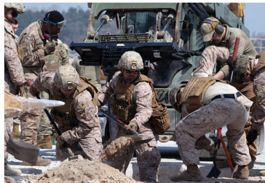
U.S. service members assigned to the 8th Civil Engineer Squadron, Marine Wing Support Squadron 174, Marine Corps Base, Hawaii and the Naval Mobile Construction Battalion, Chinhae, Naval Base, Korea, clear a crater as part of a joint-service Rapid Damage Repair training at Kunsan Air Base, Republic of Korea, March 23, 2026. RDR is critical to restoring flight line operations quickly, ensuring mission continuity by enabling aircraft to resume sorties with minimal delay after receiving damage from an attack or inclement weather ▲
