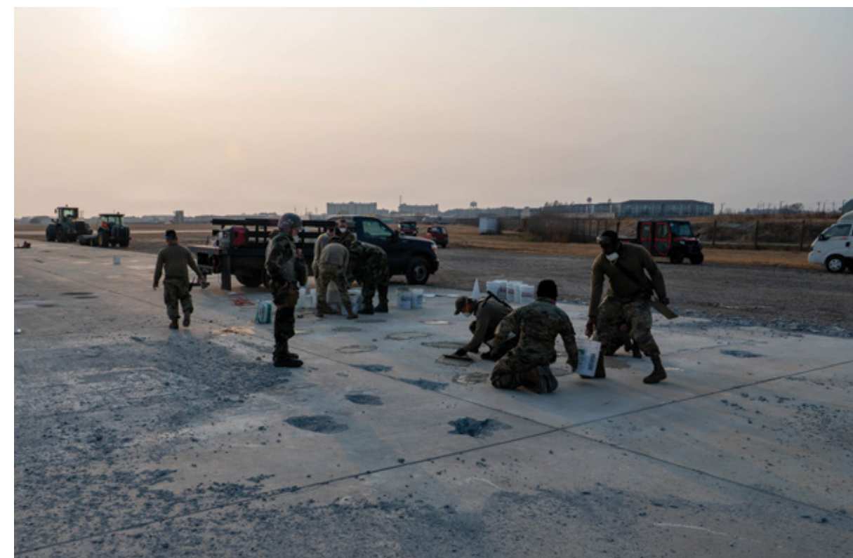
U.S. Air Force Airmen assigned to the 8th Civil Engineer Squadron conduct airfield damage repair training during exercise Freedom Shield 26 at Kunsan Air Base, Republic of Korea, March 11, 2026. Hands-on training strengthens the squadron's ability to rapidly transition from damage assessment to repair, preserving operational momentum across the airfield. ▲
