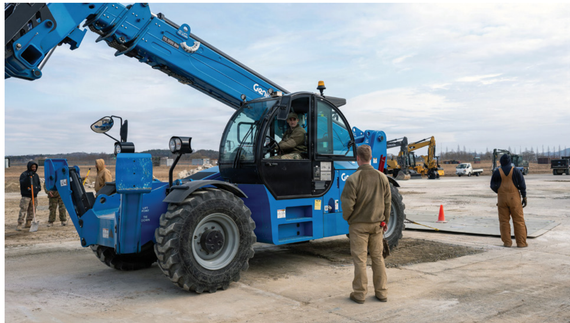
U.S. Air Force Airmen assigned to the 51st Civil Engineer Squadron pull a fiber reinforced panel during Rapid Osan Airfield Recovery training at Osan Air Base, Republic of Korea, Feb. 27, 2026. The panel-based technique is designed to rapidly return the runway to operational status in support of aircraft launch operations. ▲
